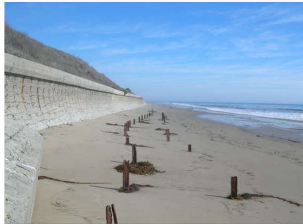
A sea wall at Arroyo Quemado beach in California. Photo credit: US National Science Foundation https://www.nsf.gov/news/mmg/mmg_disp.jsp?mediaid=72364&from=
